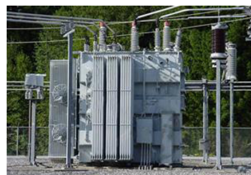
Step-up transformers increase the voltage from the generators at a power station for transmission over high-voltage cables in the Grid.
